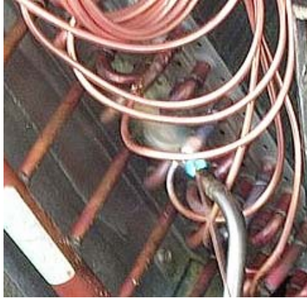
Figure 9. Brazing distribution tubes
