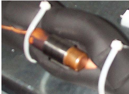
Figure 3. TXV sensing bulb clipped into place
