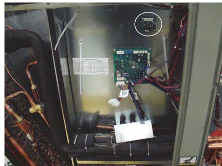
Figure 1. MMC board in D cabinet
