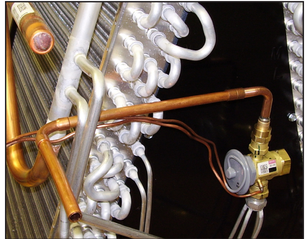
Figure 11 - Field fabricated liquid line
