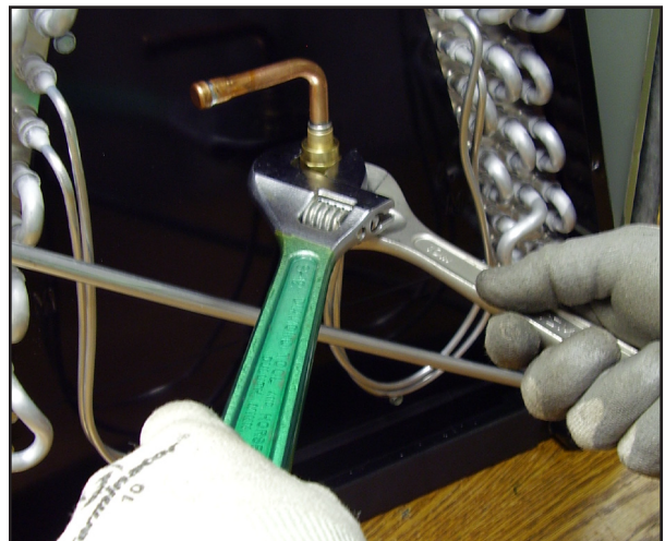
Figure 3 - Using a backup wrench
