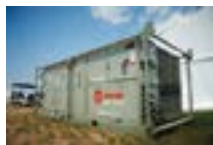
AC Units and Heaters
