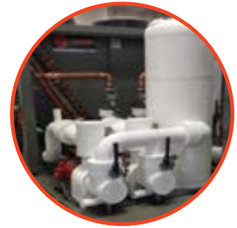
Waterside Economizer with System Pumps and Load Tank
