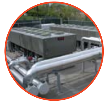
Waterside Economizer on Underground Data Center Site
