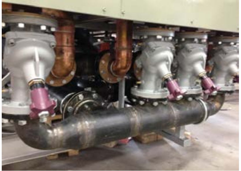
Balancing Valve per Coil to Ensure Optimal Flow
