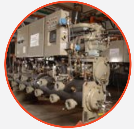
Test chiller, Trane Laboratory
