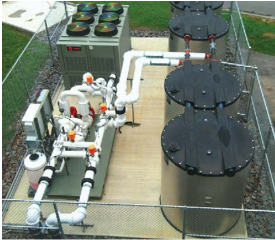
ICE System Completion module for a CGAM090 with (4) Calmac Ice Storage Tanks, dual pumps, air separator, expansion tank, glycol makeup unit, valves, and UC600 controls for variable primary operation.
