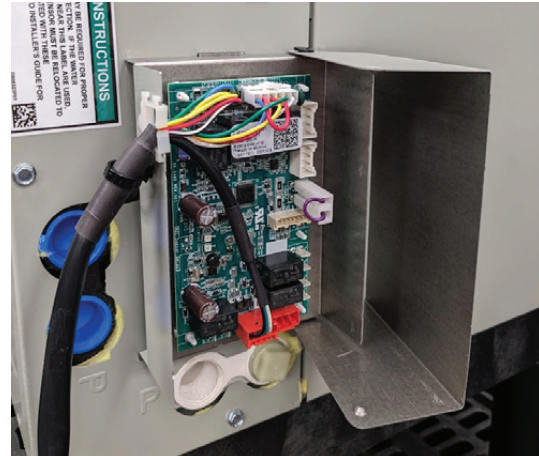
Figure 13. Coil 1 MCB control box (cover open)
