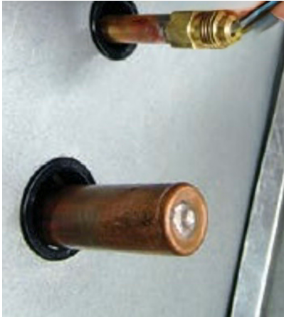
Figure 28. Nitrogen holding charge
