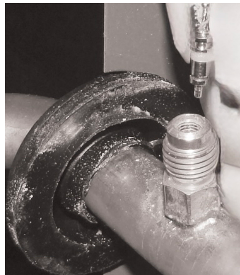
Figure 26. Valve stem removal
