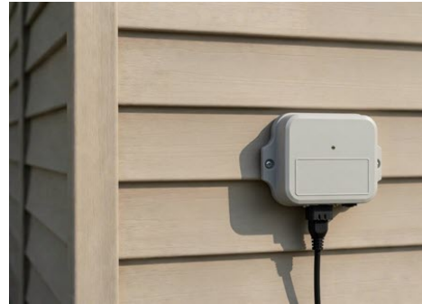
Figure 20. Mounted outdoor module
