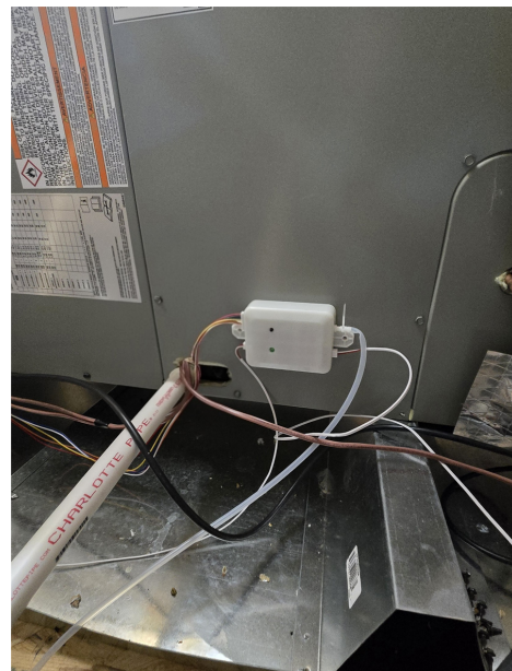
Figure 21. Indoor Module installed
