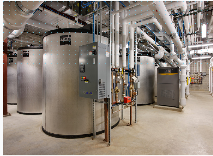
Harness the thermal energy in ice storage tanks
