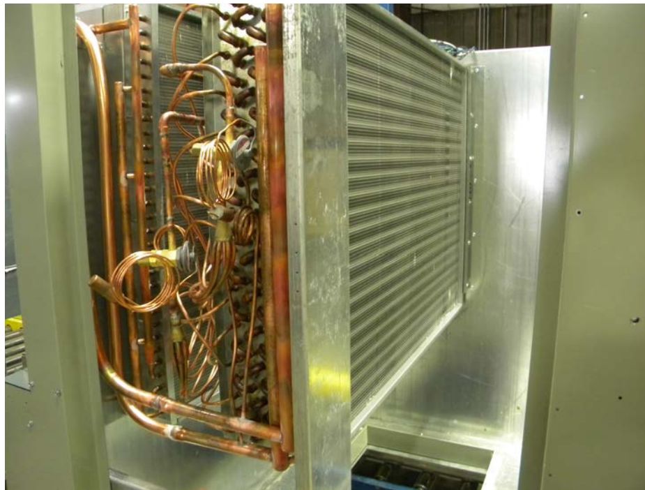
Figure 79. Evaporator and reheat coil
