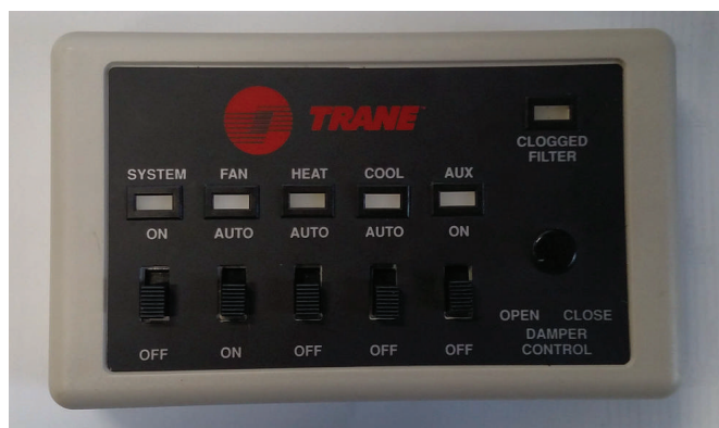
Figure 32. Remote control panel
