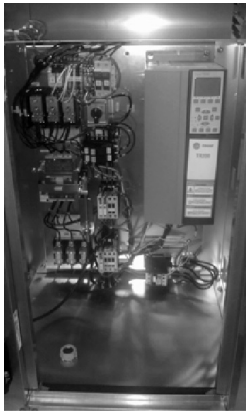
Figure 2. Integral controls cabinet for starters, variable frequency drives, and unit controllers
