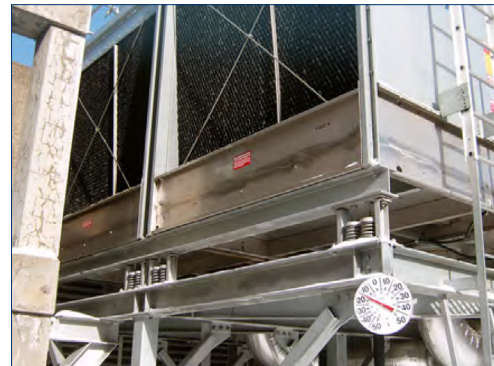
Cooling tower operating during freezing conditions
