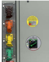
Figure 4. Main power connections and disconnect switch
