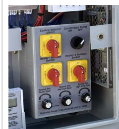
Figure 5. Condenser fan controls
