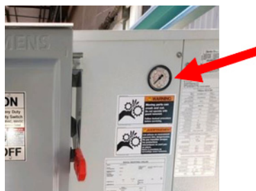
Figure 6. Unit mounted pressure gauge
