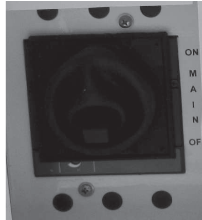
Figure 9. 50 kW and 150 kW (F0) Main Unit Disconnect
