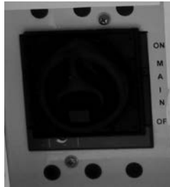
Figure 9. 50 kW and 150 kW (F0) Main Unit Disconnect
