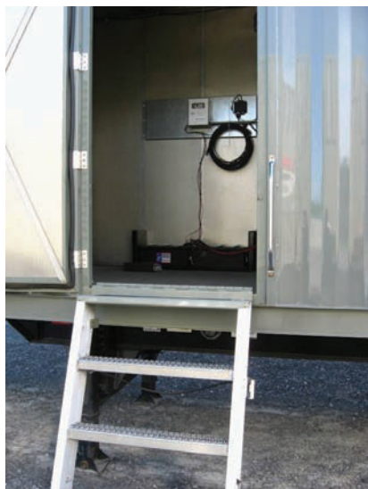
Battery Switch Access
