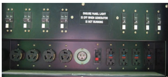
Single Phase Power Receptacles
