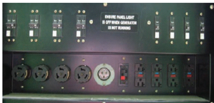
Single Phase Power Receptacles
