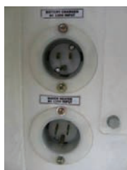
Shore Power Receptacle
