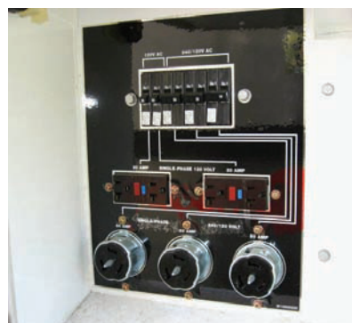
Single Phase Power Receptacles
