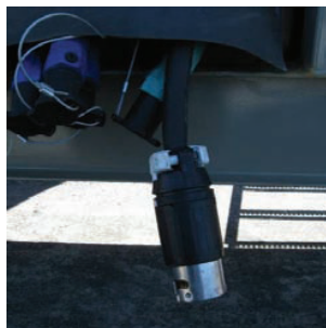
Shore Power Receptacle
