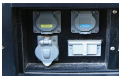
Single Phase Power Connections
