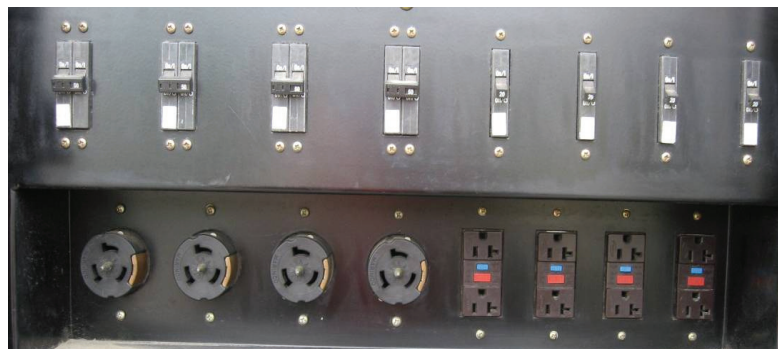
Single Phase Power Receptacles
