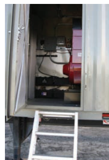
Side Door Access to Battery Switch, and Digital Controller
