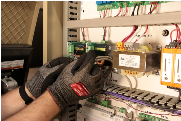
Figure 35. Power module – power cable connected to J5-1 (24Vdc+) and J5-2 (GND)
