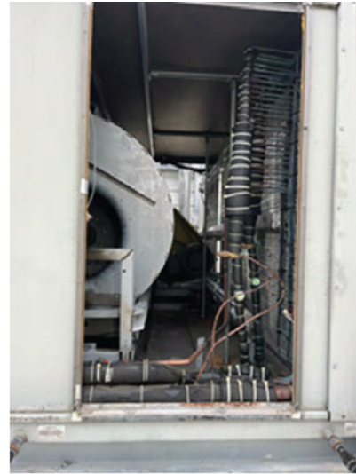
Figure 25. Supply fan (FC) motor and bearings location
