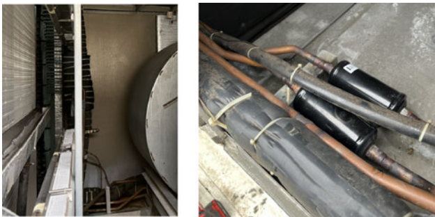
Figure 34. Expansion valves and filter driers locations
