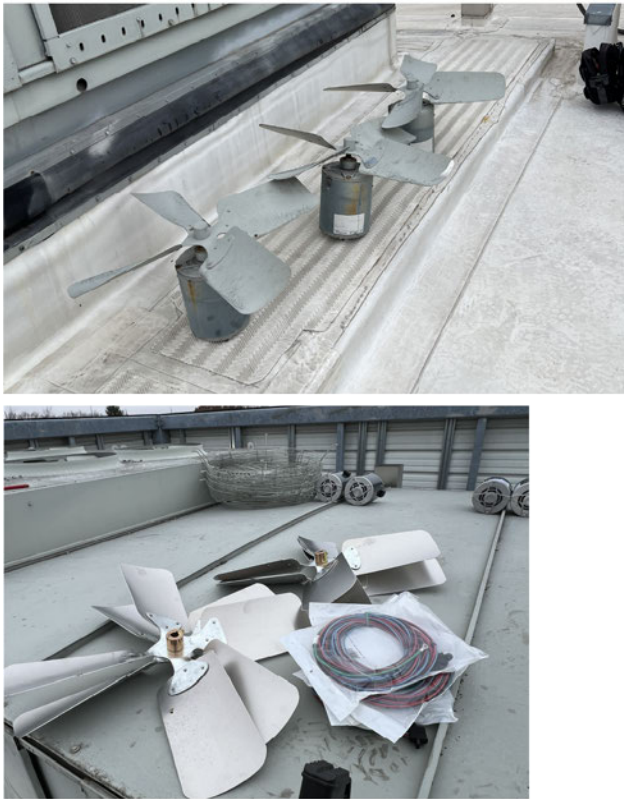
Figure 30. Condenser fan blade, motor, seal, and wire parts
