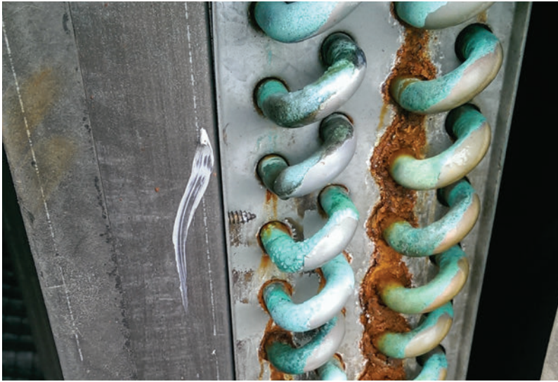
Figure 1. Major refresh option - replacing damaged coils
