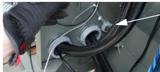
Figure 60. Route control wire conduit
