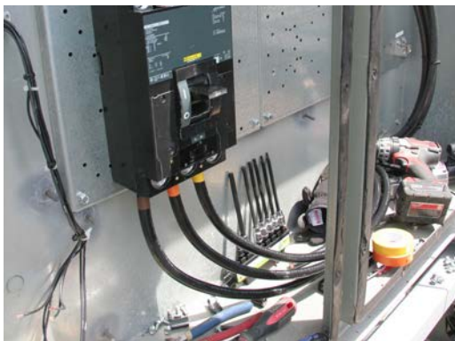
Figure 39. Load side compressor wire
