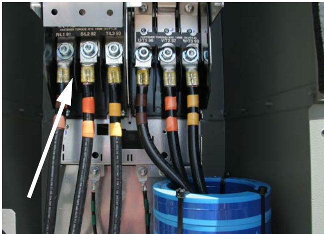
Figure 46. Load side AFD wiring
