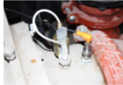
Figure 33. Flow switch in unit
