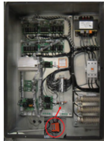
Figure 34. Monitoring module in panel
