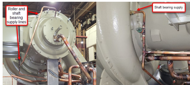
Figure 42. Oil supply lines to compressor shaft and bearings
