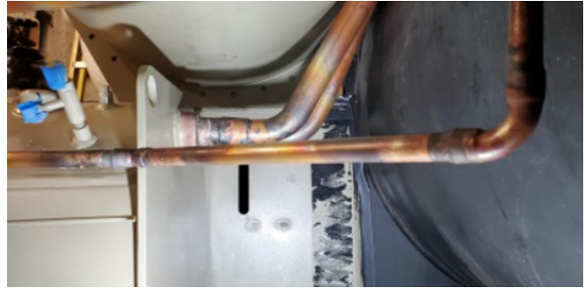
Figure 16. Evaporator vent line clearance
