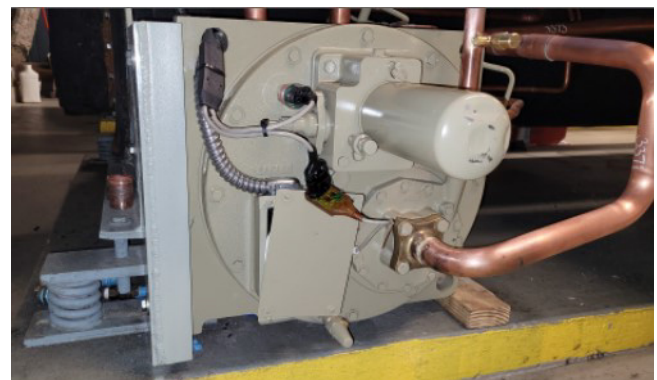
Figure 18. Oil tank elevated off the floor
