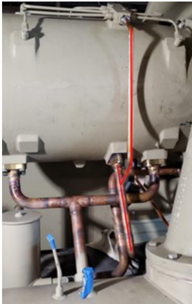
Figure 35. Refrigerant supply lines
