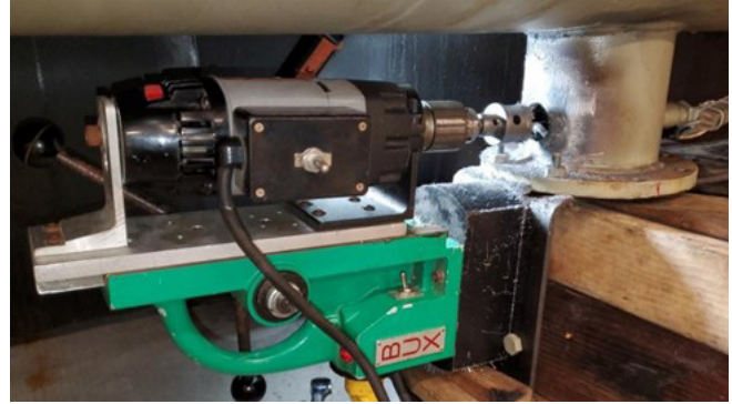
Figure 32. Drilling supply line coupling
