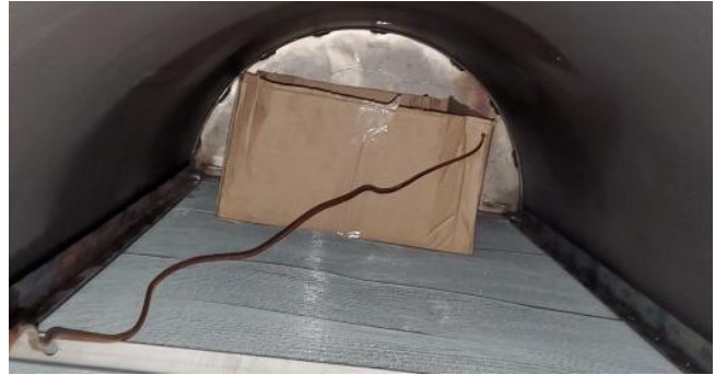
Figure 24. Box in evaporator to catch debris
