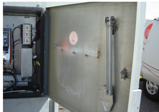
Figure 5. Fan control panel with document holder removed
