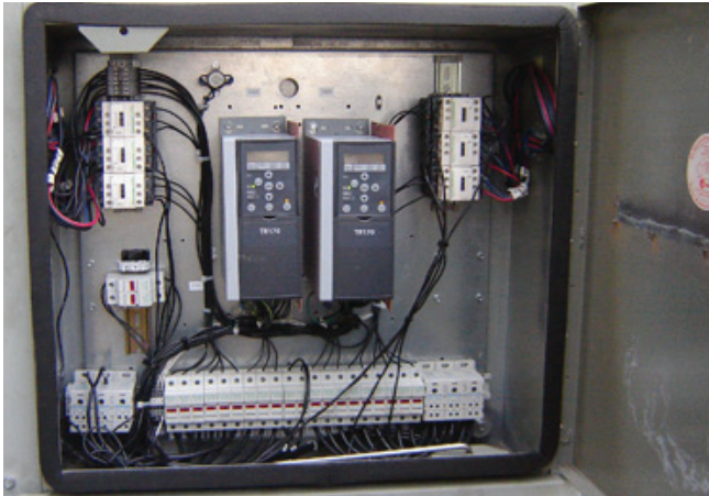
Figure 7. Mounted fan control assembly
