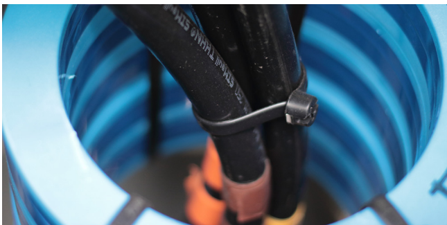
Figure 53. Wires through blue cores
