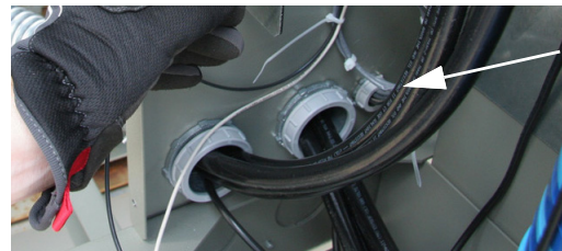
Figure 66. Route control wire conduit
