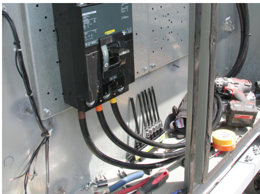
Figure 45. Load side compressor wire
