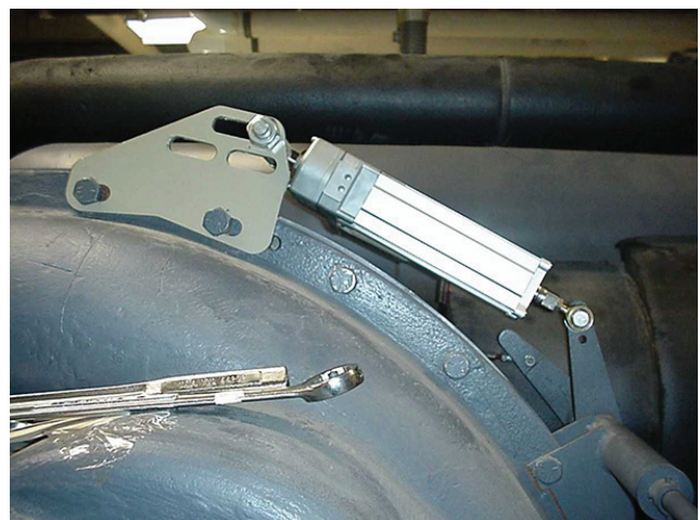
Figure 14. Installed stepper IGV actuator
