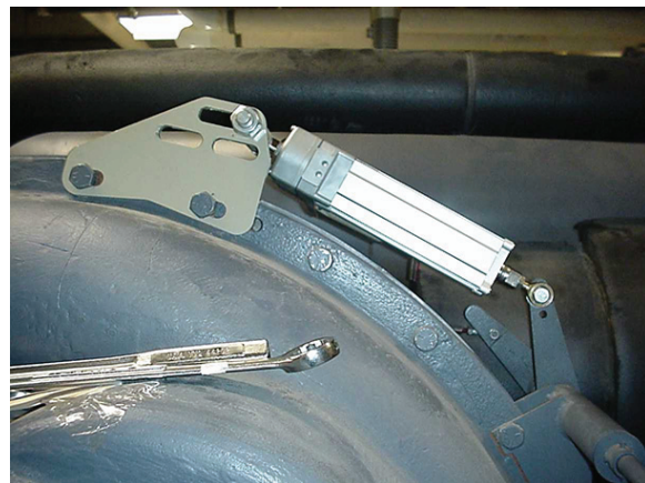
Figure 15. Installed stepper IGV actuator
