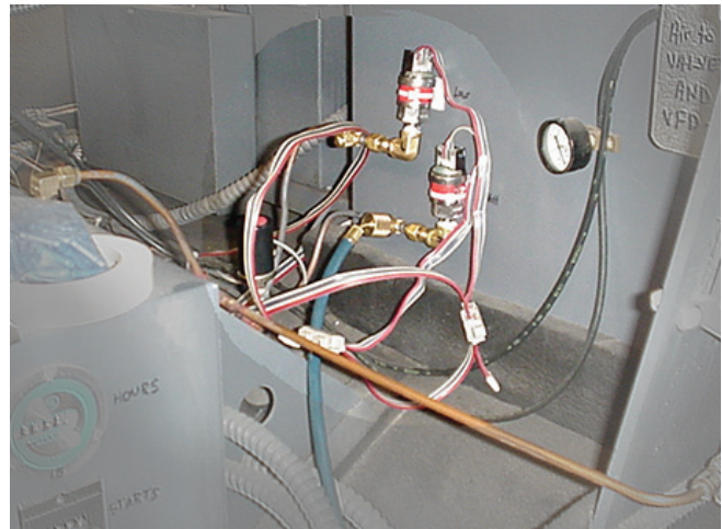
Figure 11. Pressure transducers mounted outside of control cabinet
