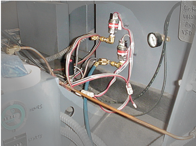
Figure 10. Pressure transducers mounted outside of control cabinet
