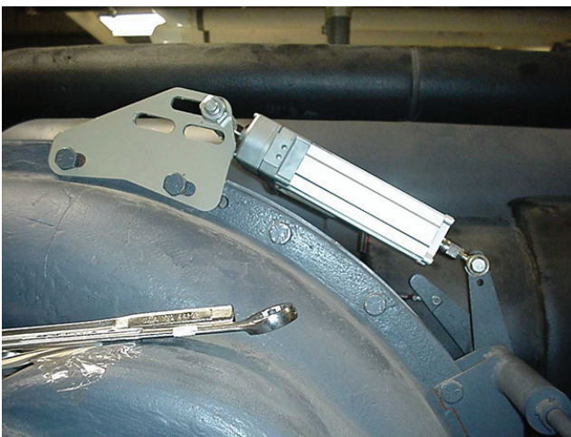
Figure 14. Installed stepper IGV actuator
