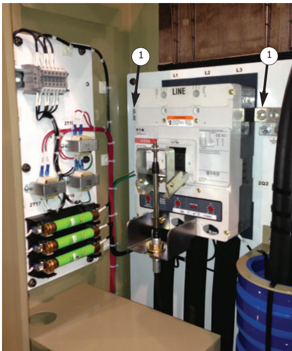
Figure 31. Location of AFDH cabinet ground terminal
