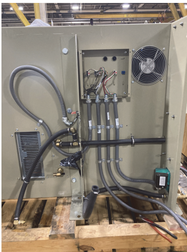
Figure 8. Glycol cooling lines
