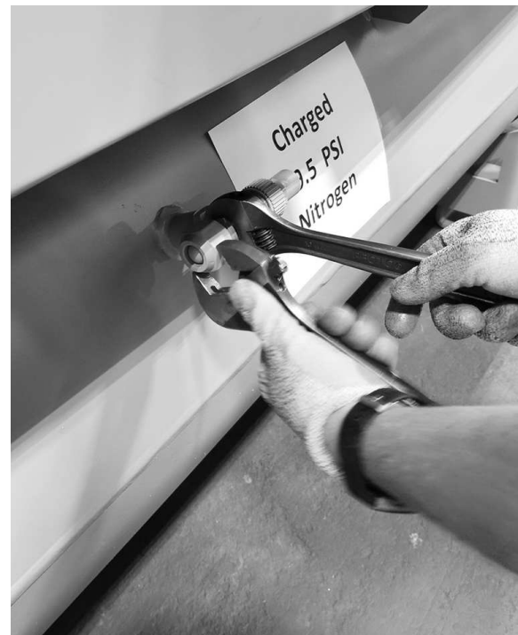
Figure 2. Heat exchanger fill valve
