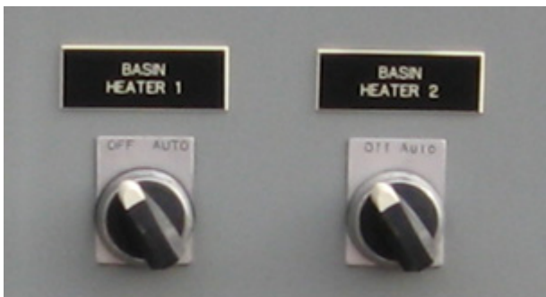
Figure 17. 500-ton cooling tower basin heater switches
