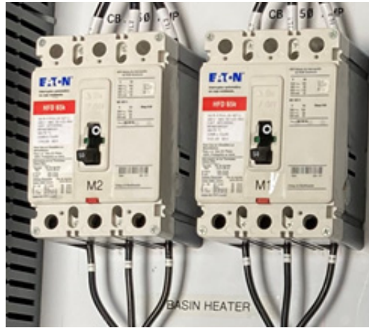
Figure 21. 1000-ton cooling tower basin heater breakers
