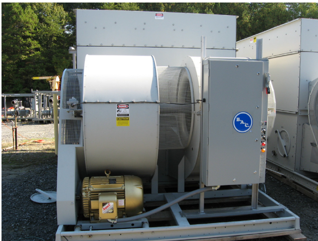
Figure 5. 270-ton CT motor control panel end
