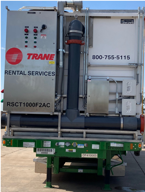
Figure 7. 1000-ton CT control panel end
