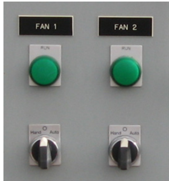
Figure 18. 500-ton cooling tower fan switch
