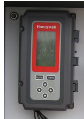
Figure 19. 500-ton cooling tower temperature control
