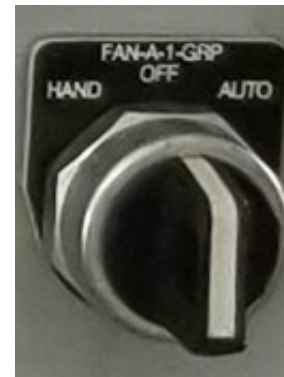
Figure 15. 270-ton cooling tower fan switch
