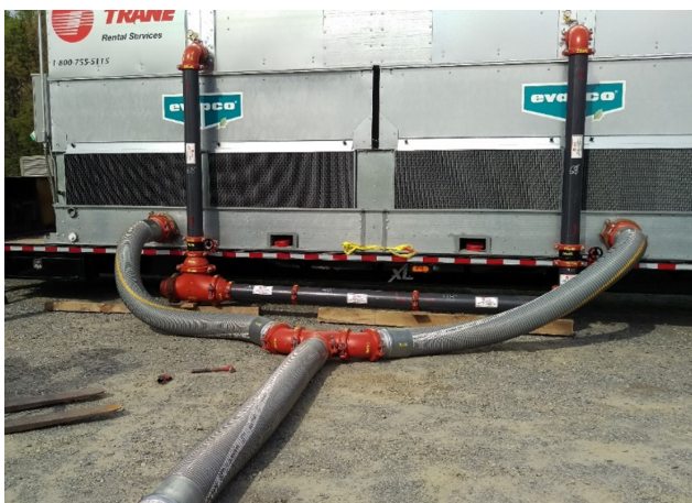
Figure 10. 500-ton cooling tower - assembled piping kit
