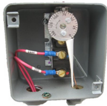
Figure 16. 270-ton cooling tower temperature control
