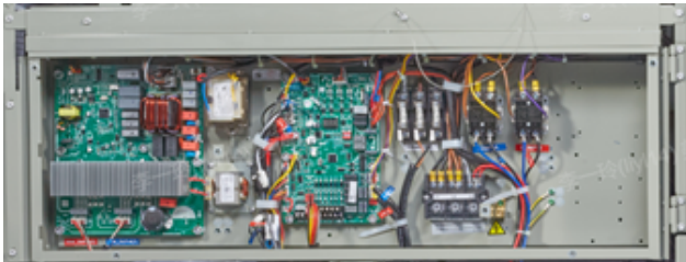
Figure 7. Low voltage control box
