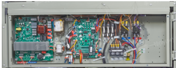
Figure 4. Low voltage control box
