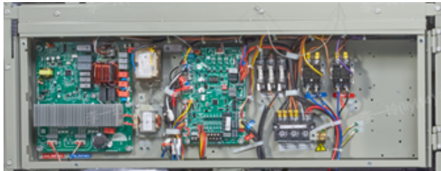
Figure 15. Low voltage control box
