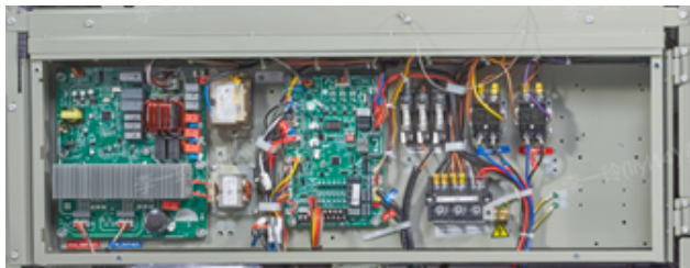
Figure 7. Low voltage control box
