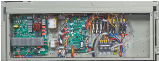
Figure 7. Low voltage control box
