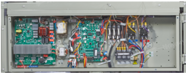
Figure 7. Low voltage control box
