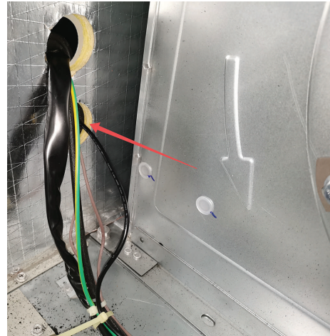
Figure 8. Supply fan blower section
