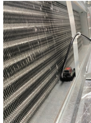
Figure 24. Moisture sensor installation and additional adhesive tape shown in cooling coil drip pan
