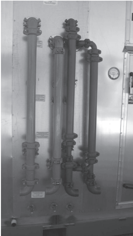
Figure 39. RSAU0050F1 piping manifold
