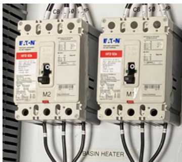
Figure 21. Cooling tower basin heater breakers
