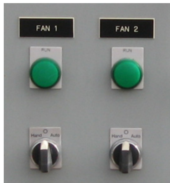
Figure 18. Cooling tower fan switch
