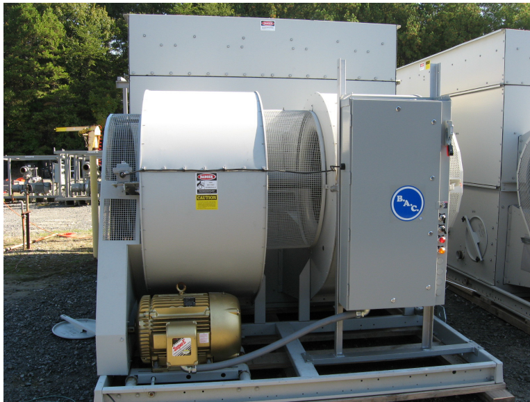
Figure 5. CT motor control panel end
