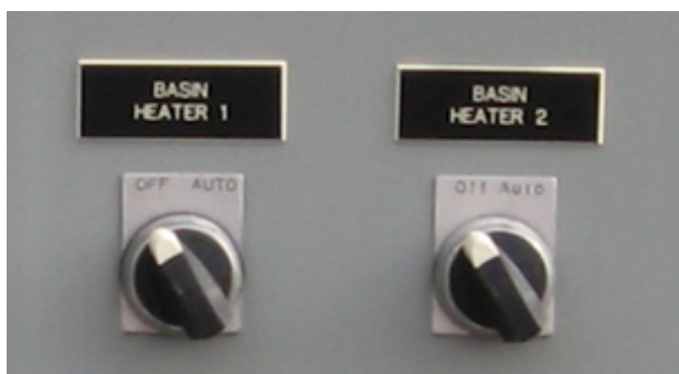
Figure 17. Cooling tower basin heater switches
