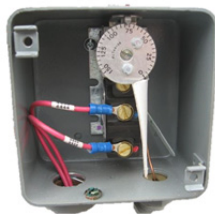
Figure 16. Cooling tower temperature control
