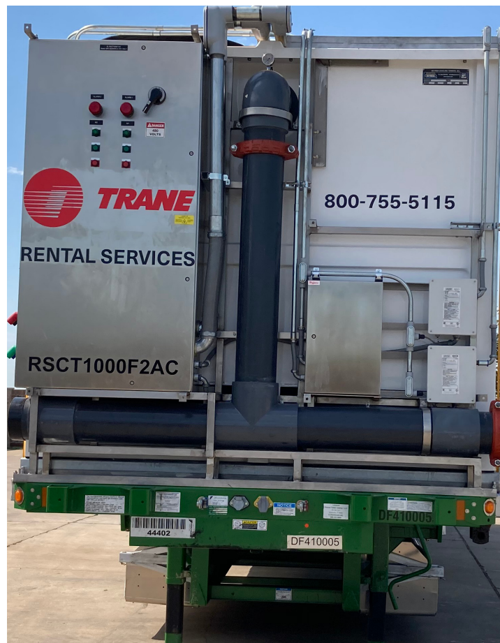
Figure 7. 1000-ton CT control panel end
