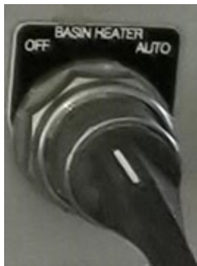
Figure 14. Cooling tower basin heater switch
