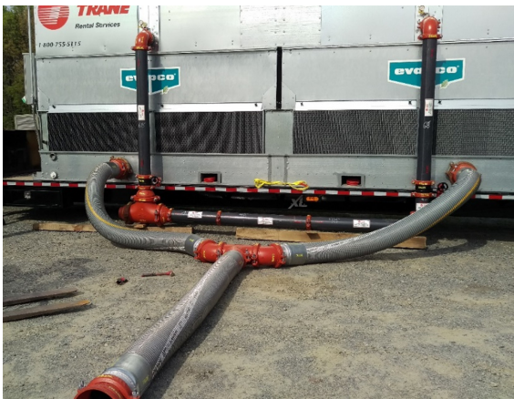
Figure 10. Cooling tower - assembled piping kit
