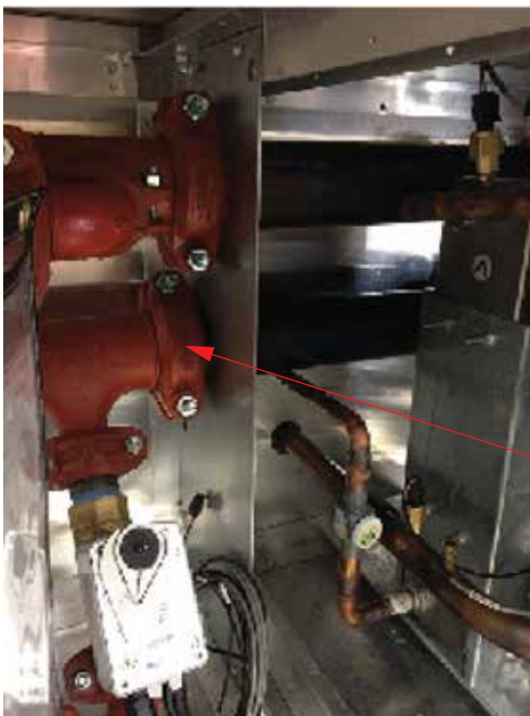
Figure 19. Condenser water bracket
