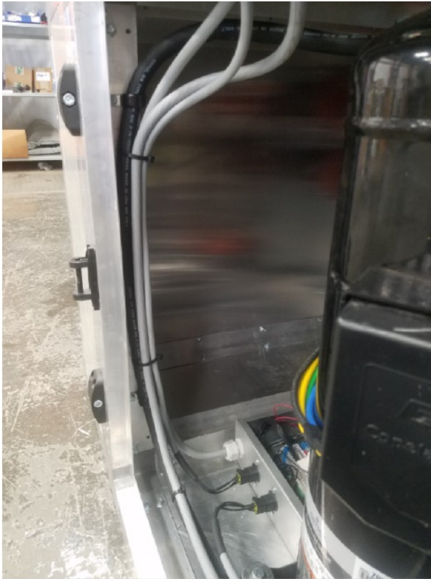
Figure 29. Fixed speed compressor power and communication wire routing
