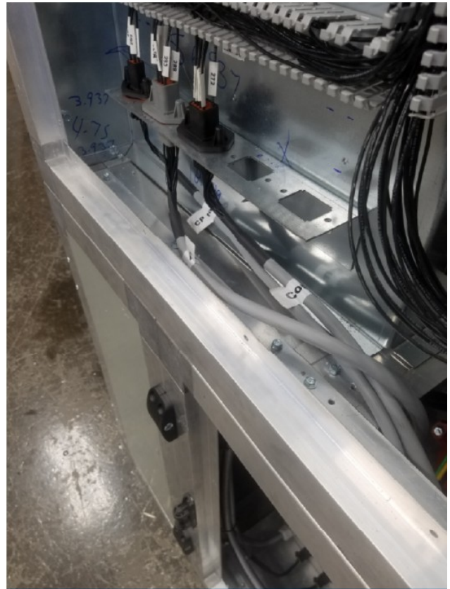
Figure 30. Compressor communication terminations
