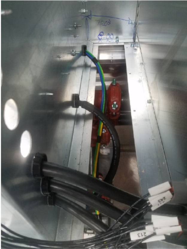
Figure 31. Compressor power wire routing to starter panel
