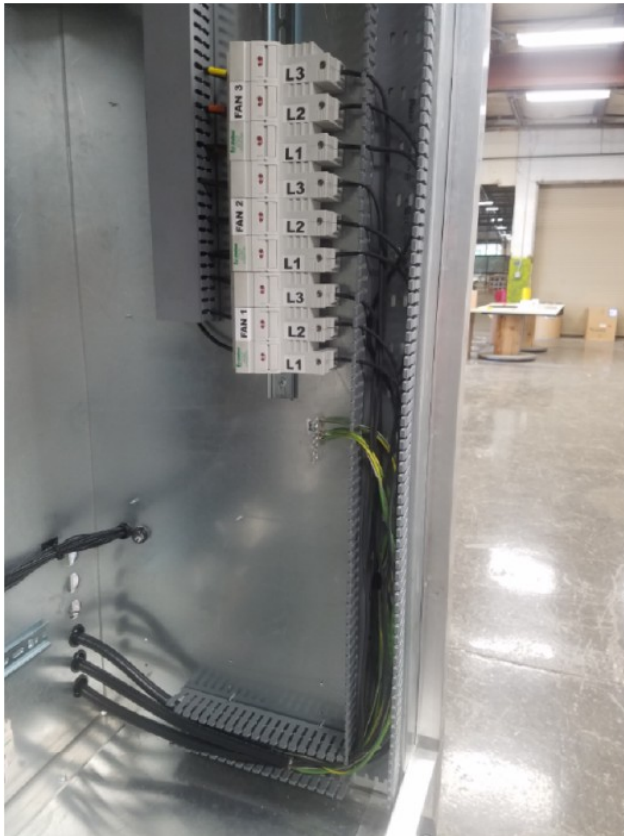
Figure 37. Fan power terminations
