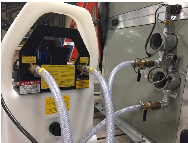
Figure 57. Rear view of Circulation pump
