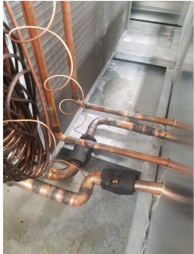
Figure 24. Braze suction and liquid lines
