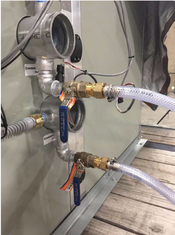
Figure 54. Typical setup for clean in place
