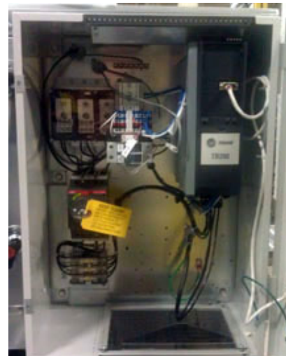
Figure 140. Externally mounted VFD
