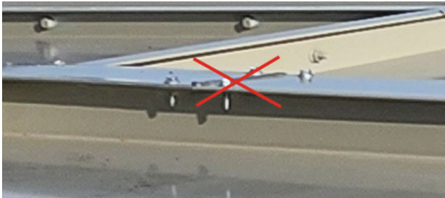
Figure 25. Do not wide roof strip
