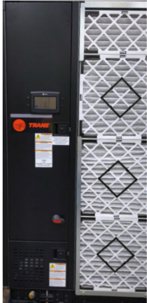
Figure 12. Electrical cabinet door
