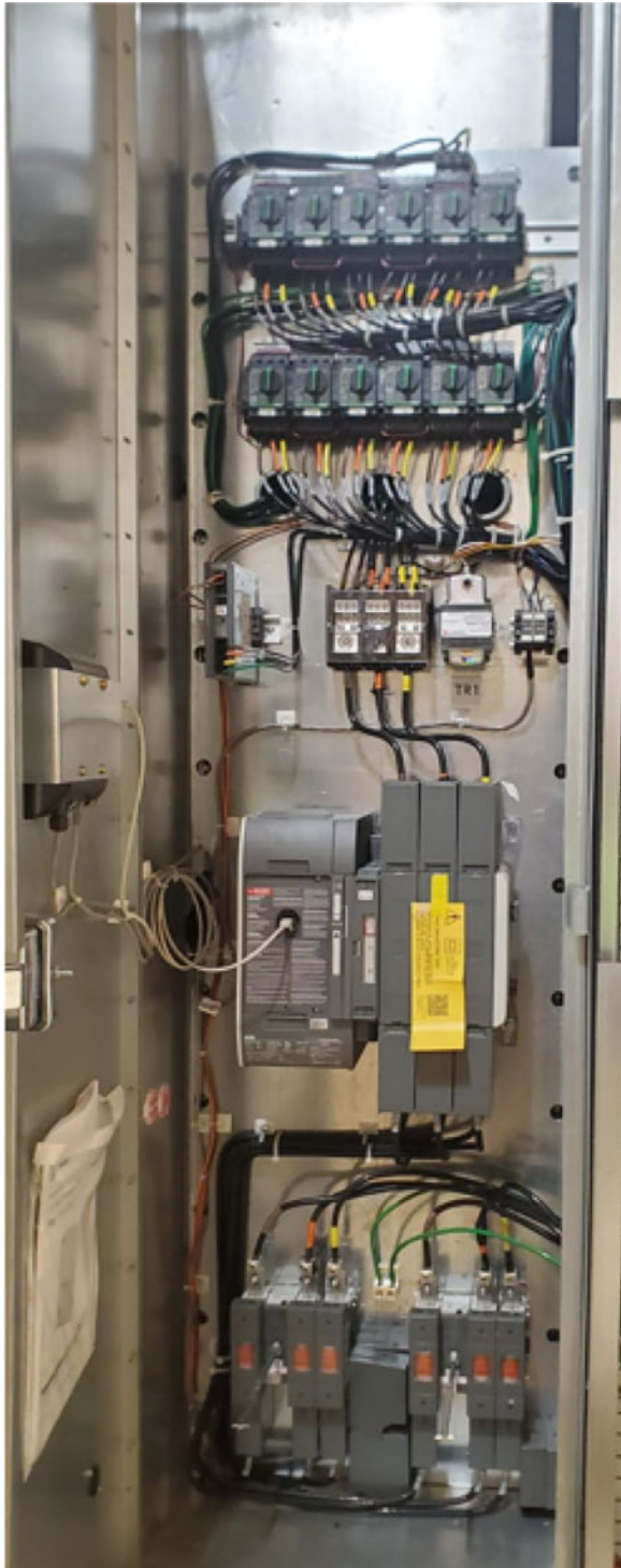
Figure 13. Typical electrical panel
