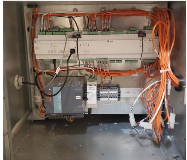
Figure 14. Low-voltage electrical panel
